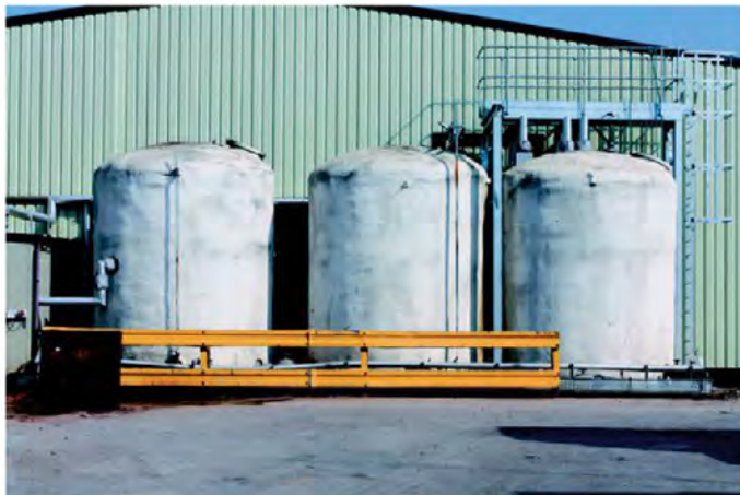
These tanks hold treated chilled water ready to be re-used in a potato handling facility using Wonderware software.
